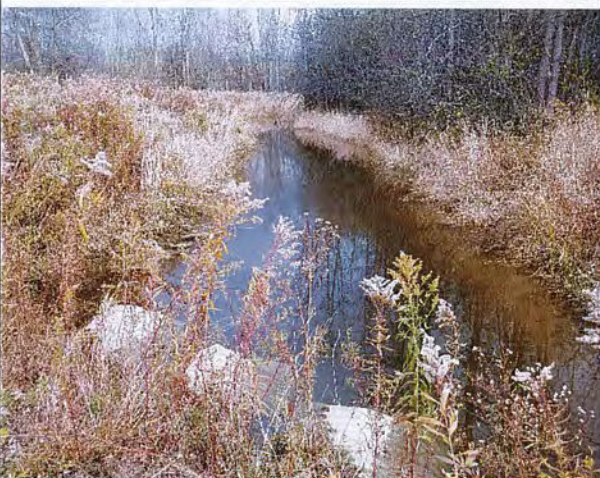
Photo 5: Crossing through drain at west side of Lot 15. Four- 1 m rise x 650 mm span structural plate corrugate steel arch culverts.
